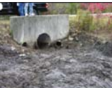
Outlet culvert to the ditch. The two side culverts were buried, and were discovered during excavation. Notice there is only a trickle of water from the large culvert. Stains on the pipe show the original level of sediment accumulation.
