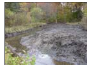
The ditch was dug to the width of the culvert. Notice how the water pools in the ditch because it is too wide for the capacity and velocity of flow from the culvert.
