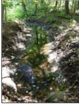
The width of the ditch is wider than necessary for the amount of water flowing into the culvert
