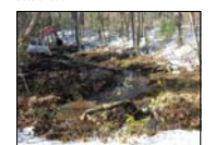
Final view of ditch from same vantage point as "before" picture. Stream will be monitored to see if it is sustainable.
